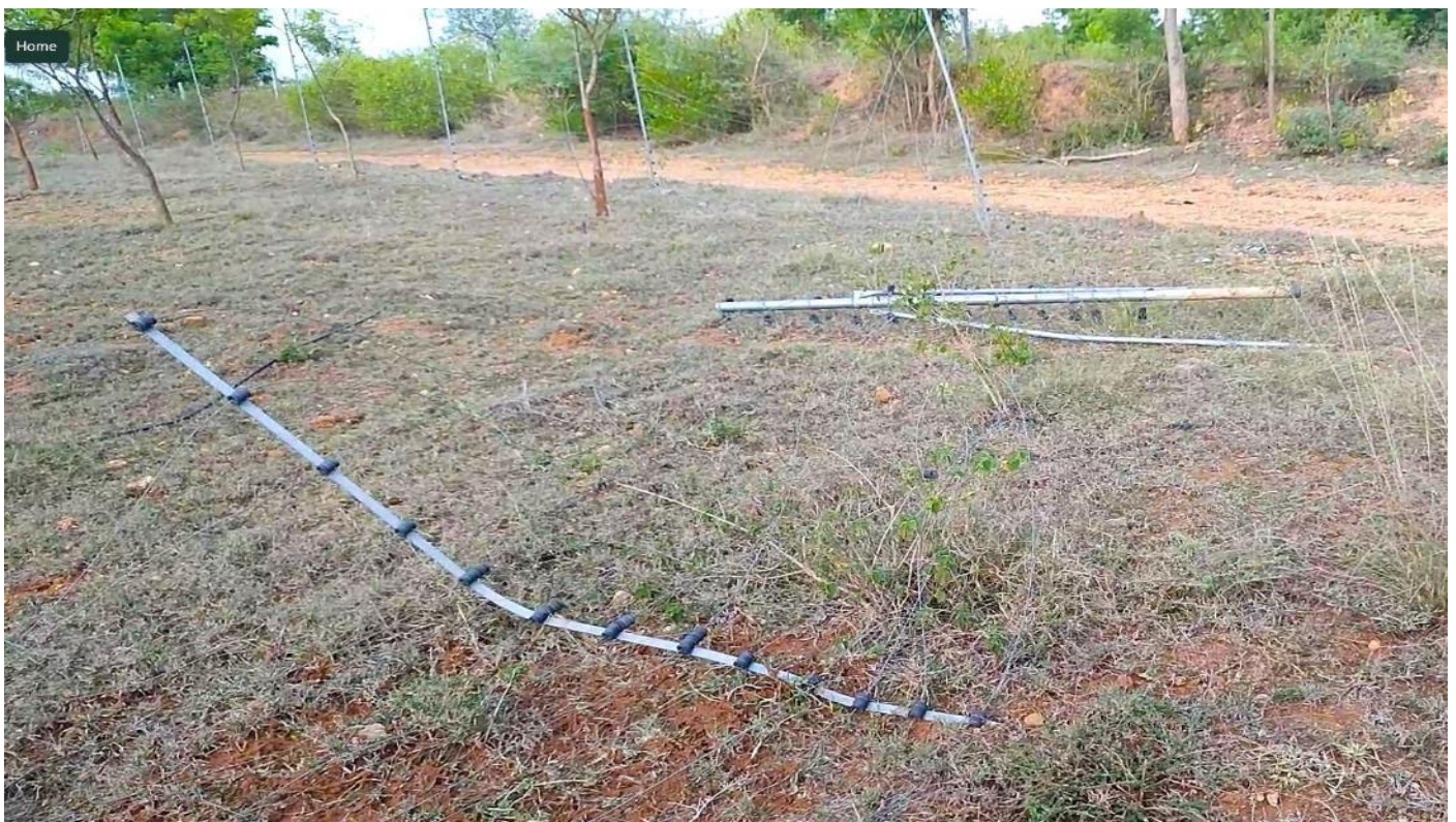
Main solar cable carrying post (on right) and supporting post (on left) damaged by elephants. Poles do NOT carry the power
